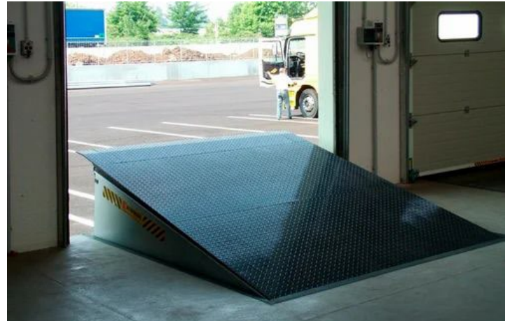
Figure 32: The dock leveler is the bridge between the truck floor and the warehouse yard
