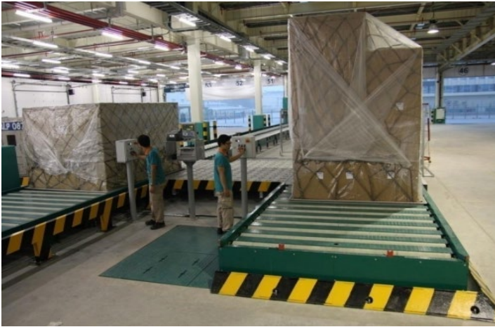
Figure 33: SCS Automated Conveyor System
