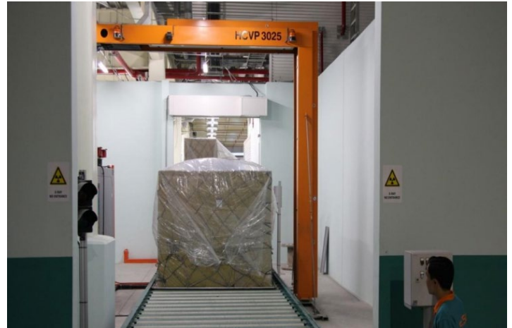
Figure 34: The X-Ray automatic scanner can handle goods with a height of 4.5m and a width of 3.2m in about 2 minutes
